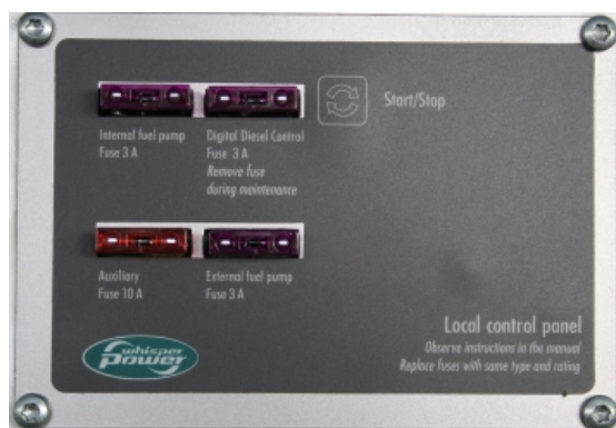
Figure 6: Local control panel
